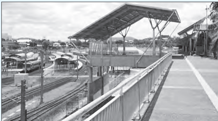
Roma Street redevelopment Package 31 – one of the shade canopies in the package incorporating roof truss structure, offices, aggregate and structural steel shade canopies.
